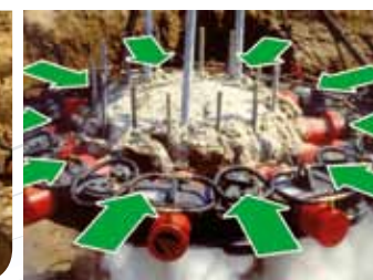
The release of the chisels allows the pile to be uniformly cropped.
