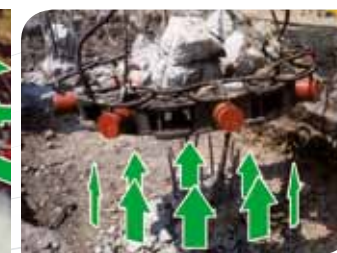
Once the pile has been demolished by lifting the Pile Breaker it keeps hold of the material freeing it from the reinforced structure.
