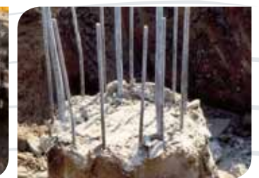
The final result is the perfect cleaning of the reinforced structure while the structure of the pile remains unchanged without creating cracks on the lower part which is still below ground.
